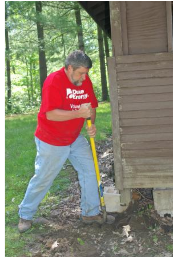
Duke Energy's Steve Welte of Fairfield raised the foundation of a chalet at Timber Hill camp in Fairfield Township. About 20 members of Duke's information technology department in downtown and Plainfield, Indiana worked at the camp May 19. Sue Kiesewetter/for the Enquirer
